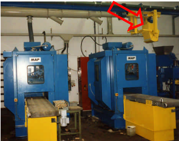
Pic. 1: Core sand feed by hoist gear system (arrow) to core shooters
