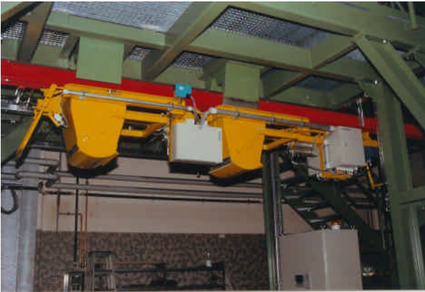
Pic. 3: Hoist gear with two buckets, charging from an upper mixer level
